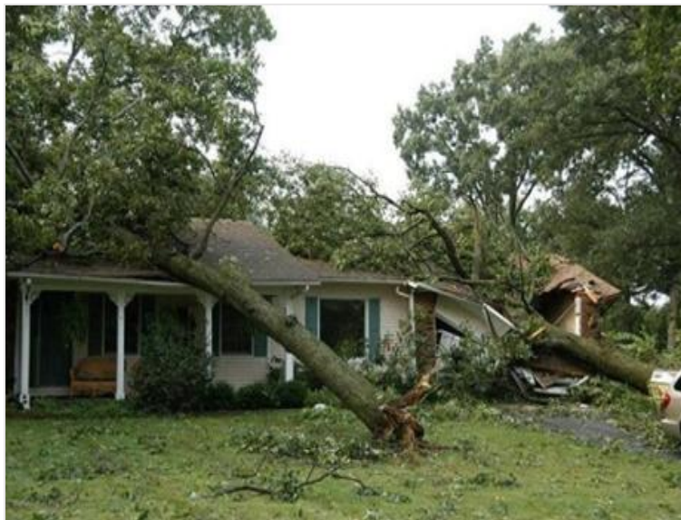
Figure 40: Home Damaged During Windstorm
