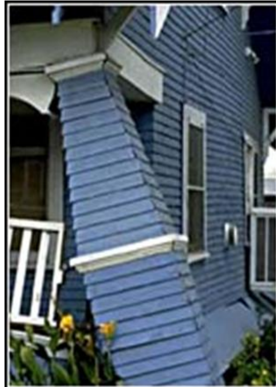
Figure 27 Structural Earthquake Damage
